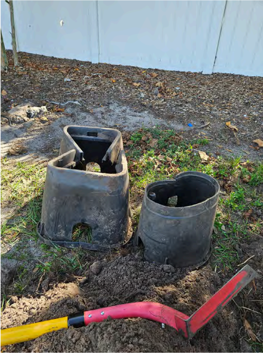
Damaged valve boxes
